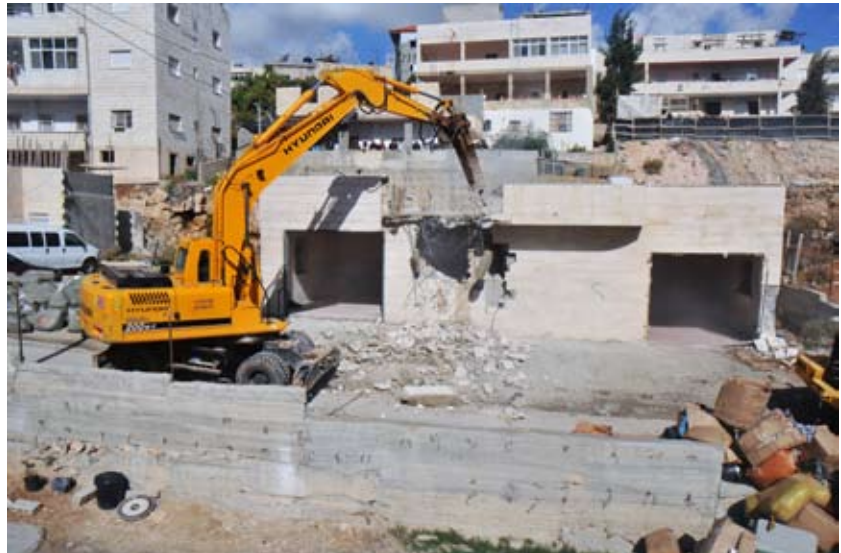
House Demolition in Al Esawiya, East Jerusalem. Photo by Mahmoud Yllayan, November 2009
