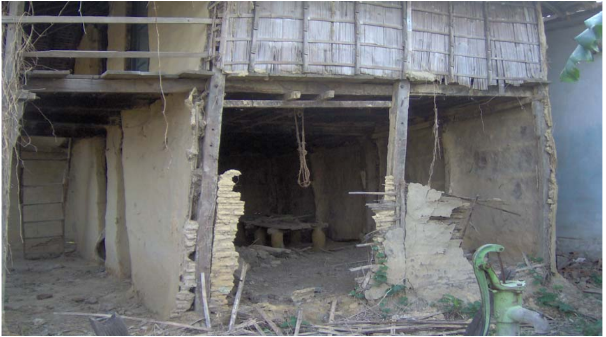
Destroyed House by Security in Dhanusadham VDC, Dhanusha.
