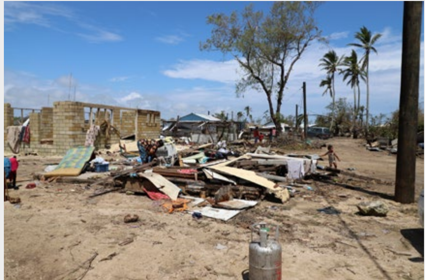
One of the many houses that have been completely destroyed by Tropical Cyclone Gita after it hit Tonga's main island. Photo: IFRC/Gemma Snowdon, February 2018
